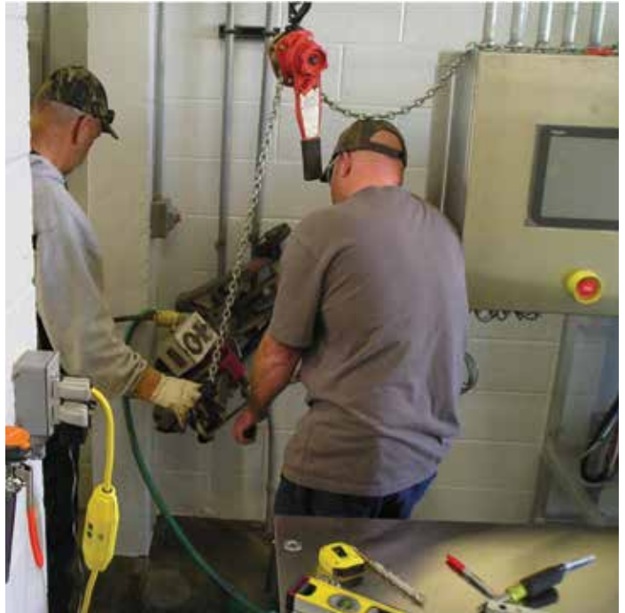
After reviewing their options, Vacaville staff ultimately opted to purchase a 400-lb/d on-site sodium hypochlorite system (below). They installed the system themselves in early 2014 (right).
