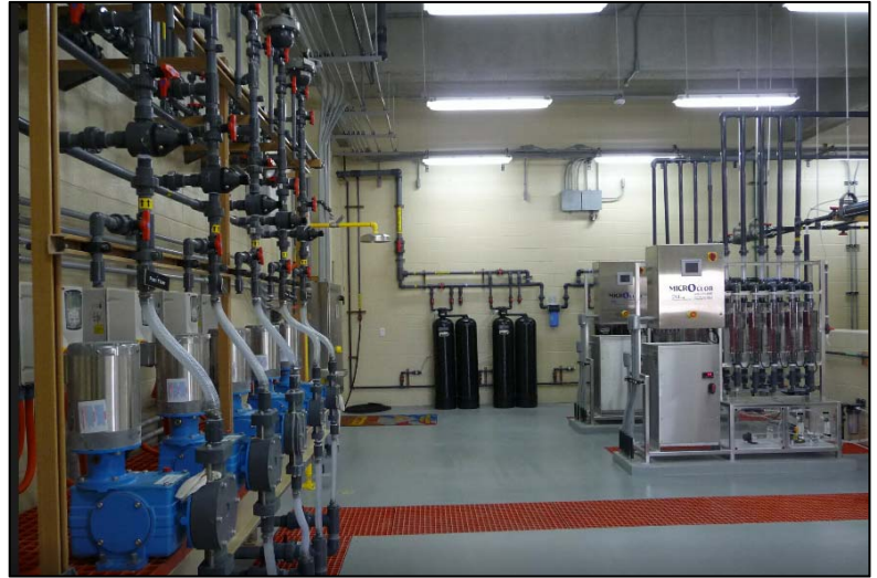
Microclor™ OSHG systems with Encore® metering pumps in foreground
