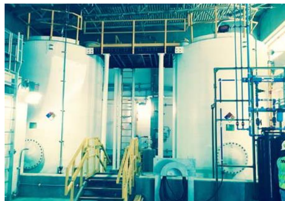
Hypochlorite (Bleach) Storage Tanks
